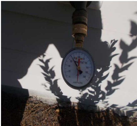
Water pressure was a steady 60+ PSI
