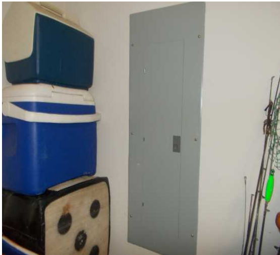
Main panel box.
