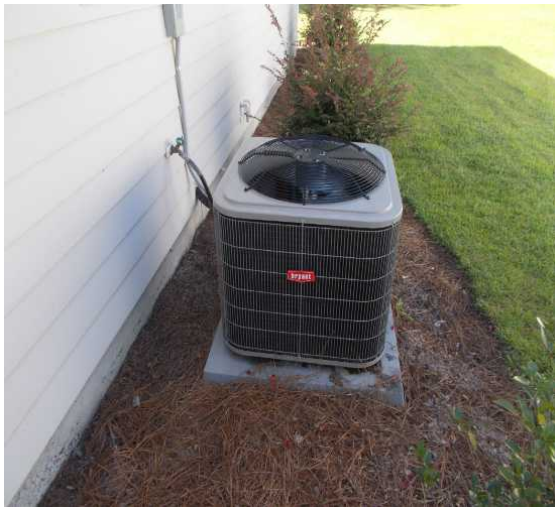
Heat pump at the right side of the home.
